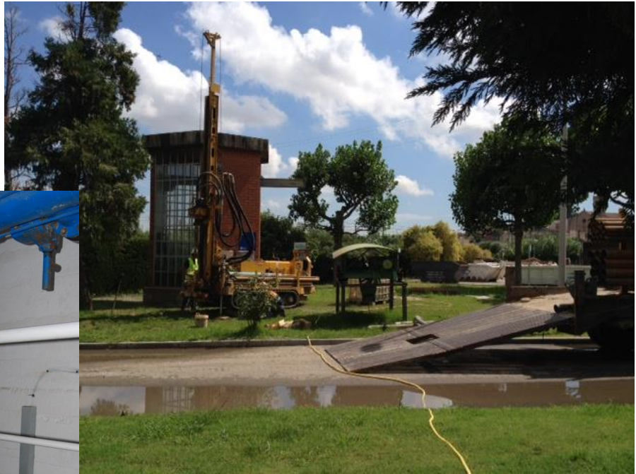
Figure 5 Llobregat pilot site in Barcelona, injection system (left) and drilling works (top)
