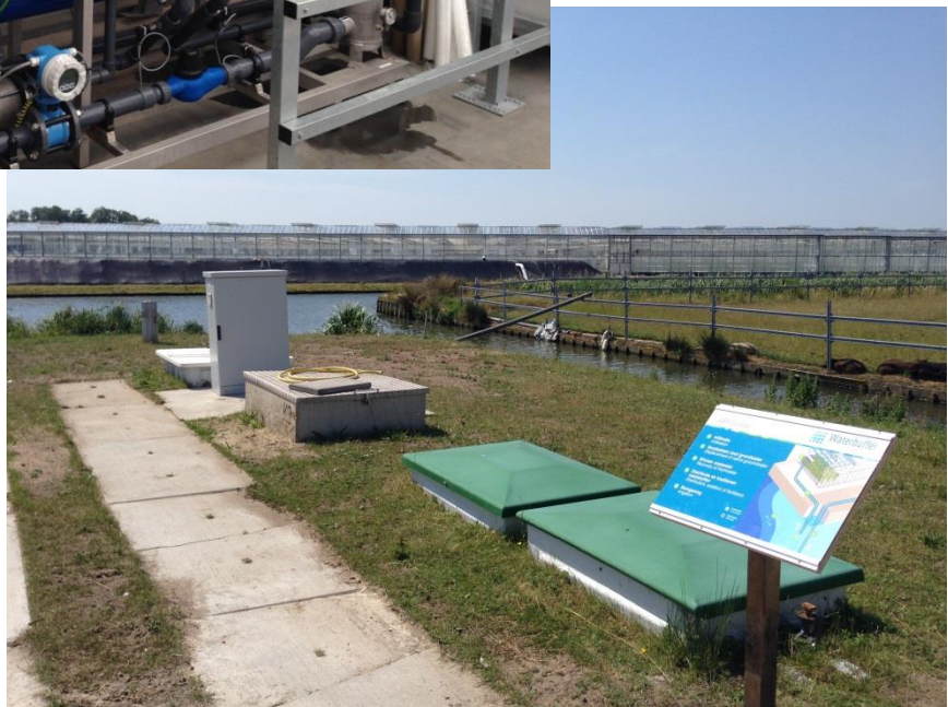
Figure 3 The Westland setup with the Reverse Osmosis system (top) and infiltration / recovery system (below)
